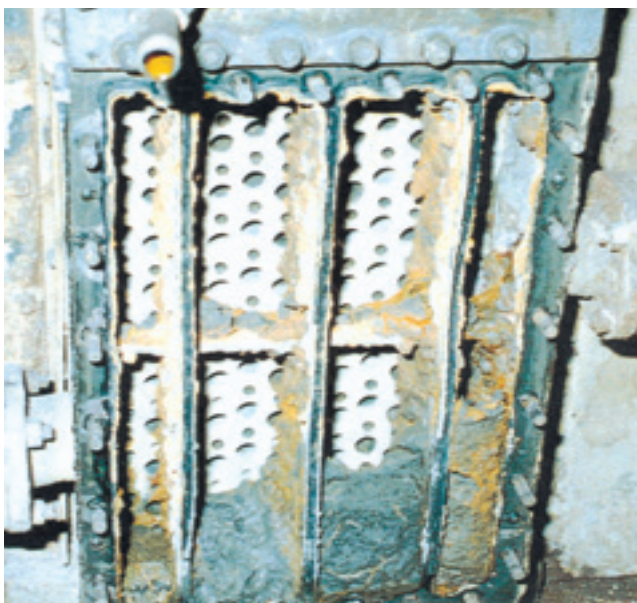
Fig. 12 — Heat exchanger after one year of service.
