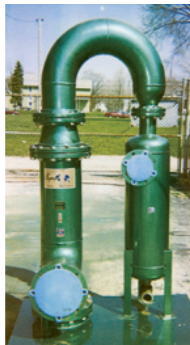
Fig. 9 — Magnetic water conditioning installation.
